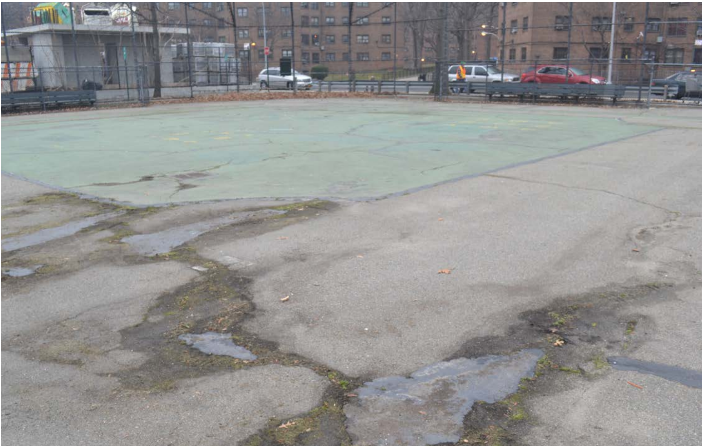
Water damage erodes the play surfaces at Hallet's Cove Park in Astoria.
